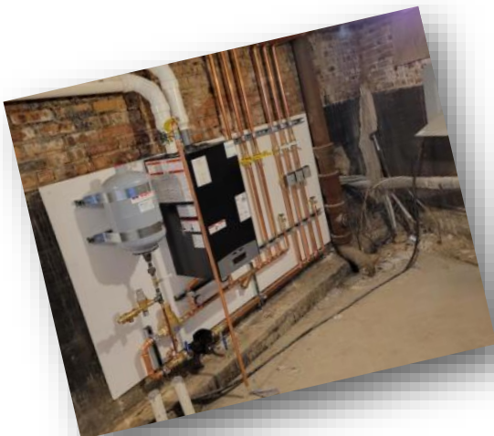
COMPLETED BOILER FOR RADIANT HEAT IN THE CHURCH
