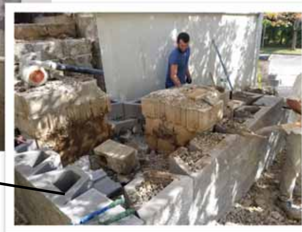
Rotten Wall Sheathing
