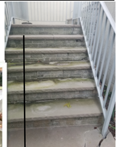
Dangerous Condition of Steps
